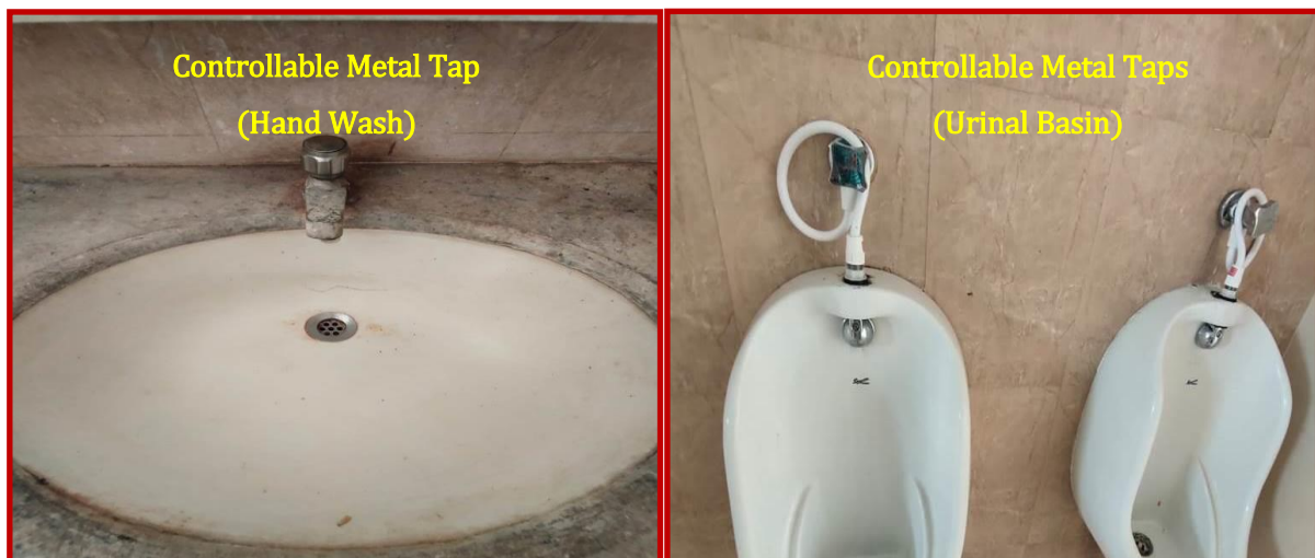
Fig.4: Different Types of Taps used in Water Distribution Network
