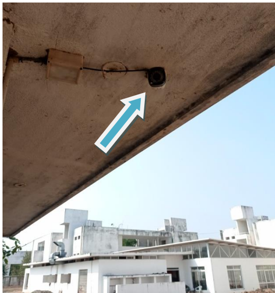
CCTV Camera Installed at Boys Hostel Entrance
