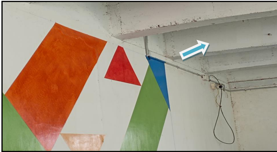
Camera Installed at Students Corner (lunch Hall)
