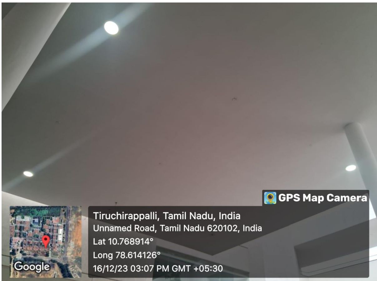
Fig. 7.1.2.4 LED Lights in corridors
